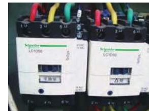
schneider AC contactor
