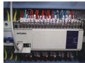
Mitsubishi PLC control Unit
